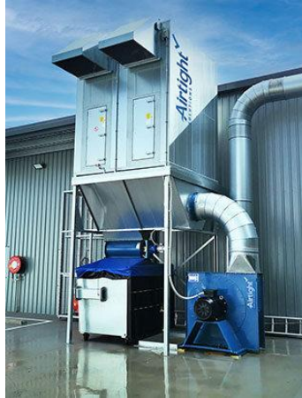
Dust collector & extraction systems
