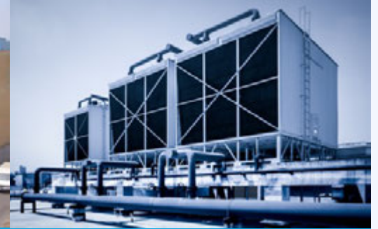
Heating and Cooling Systems
