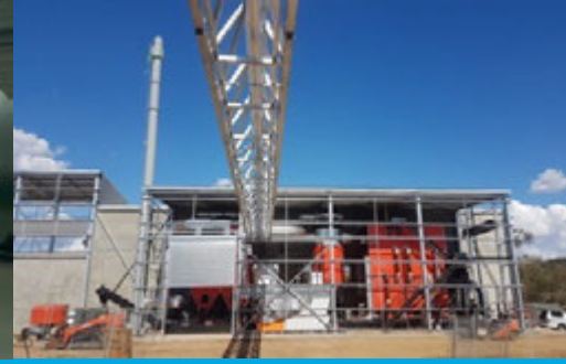
Biomass Steam and Hot Water Generation
