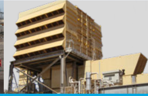
Inlet Filter Houses
