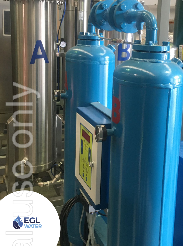
Charged Gas Generation Equipment
