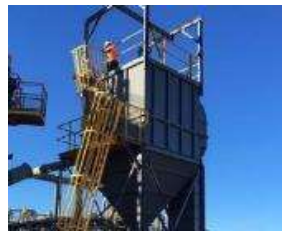
Fabric Filter (Baghouse)
