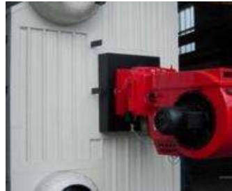
Industrial Steam Boiler
