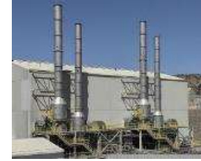
Particulate Scrubber / Cyclones
