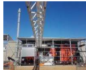
Biomass Steam & Hot Water Generation
