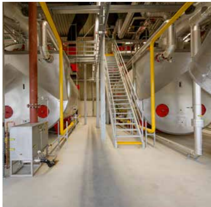
Flue gas heat exchanger ECO 1
