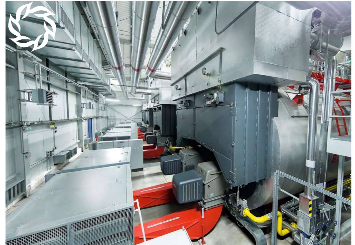
The superheater modules are installed on the front reversing chamber of the boilers.
