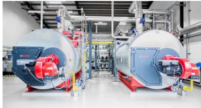
The two efficient Bosch steam boilers supply a total of up to 8 t/h of steam.
