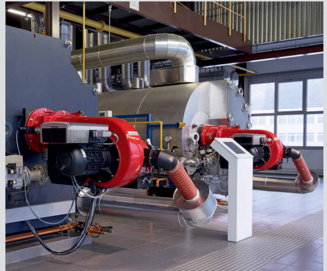
Burners with FGR on long-term test in the Weishaupt factory's boiler room
