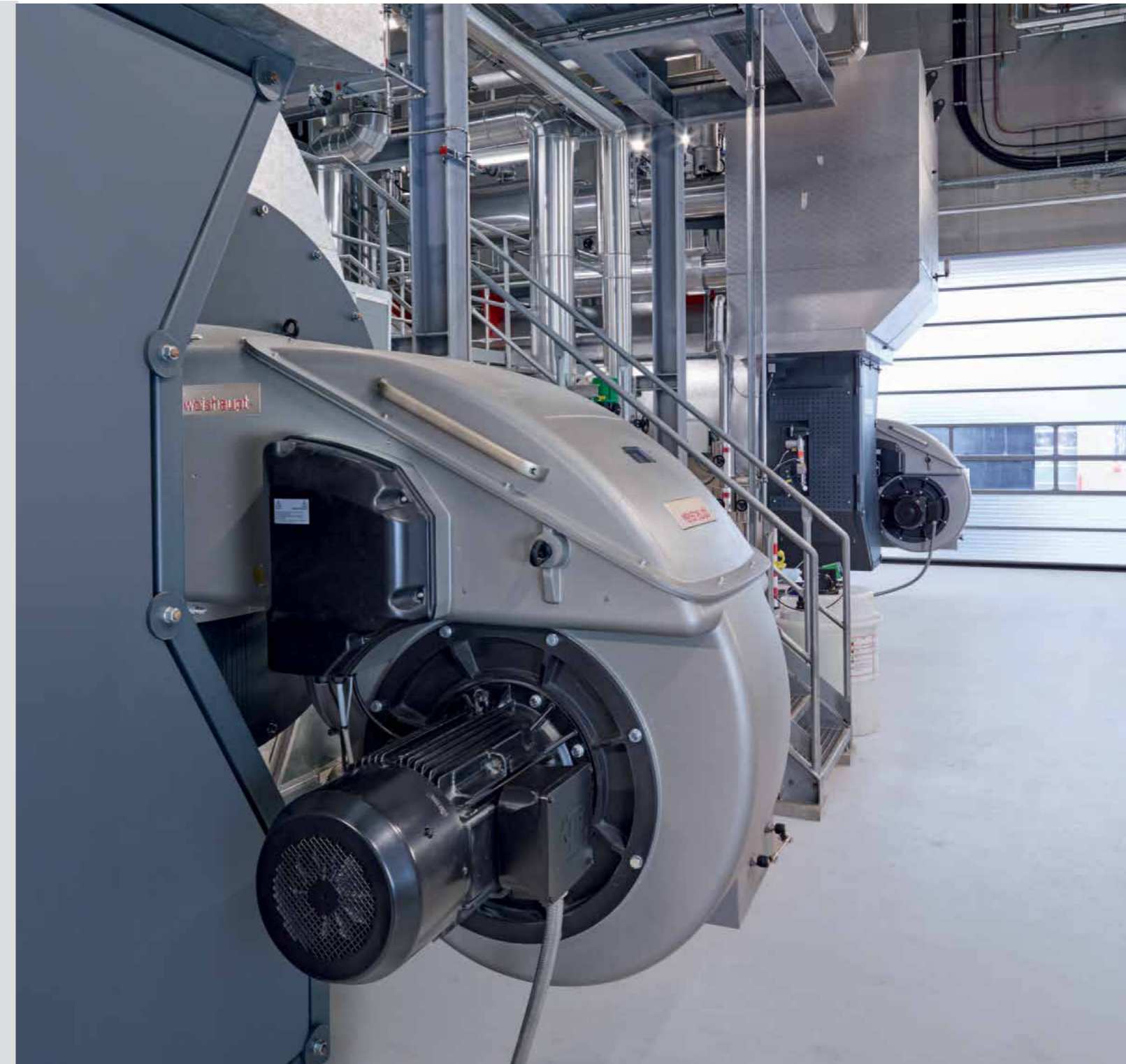
Heat supply at an industrial premises (total steam generation: 37.4 t/h)
