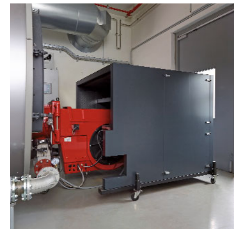
W-SH 20 in a district heating centre, with bespoke shroud cutouts for the fuel and power supplies.
