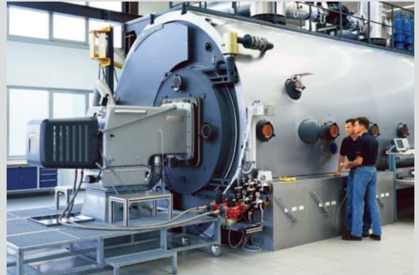
Burners rated up to 32 MW are tested on the world's largest test firing chamber in the R&D Centre
