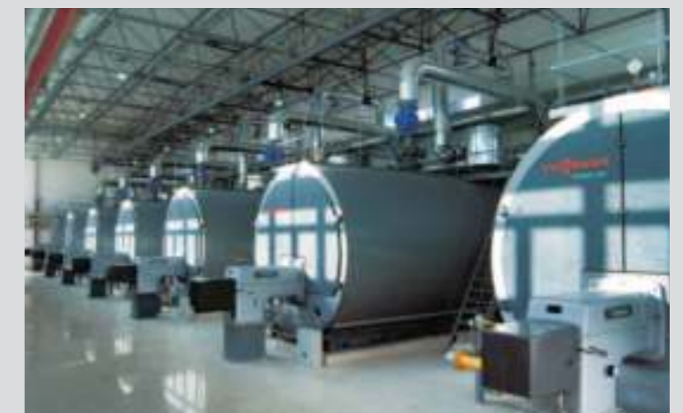
Xi'an, central China: The seven WKG gas burners in this heating centre provide more than 50 000 residents in the Zi Wei garden district with 115 MW of heat
