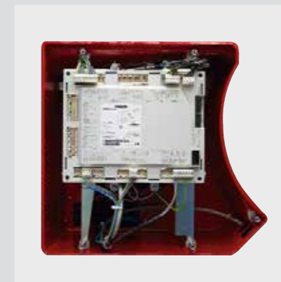
W-FM 100 or W-FM 200 combustion manager mounted in the burner
