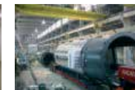
Thermal oil heater used to heat a plant for producing particleboard near Moscow, Russia, with a capacity of 12 MW
