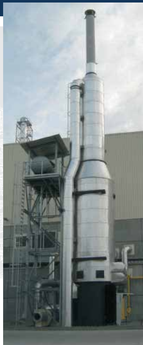
Heater in up-firing layout, capacity: 9.6 MW with built-in combustion air preheater and subsequent stack, total height: 25 m, heating of a particle-board press (Romania)
