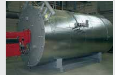
Thermal oil heater fired with natural gas with a capacity of 1.6 MW, installed in Texas, USA, application in the food industry
