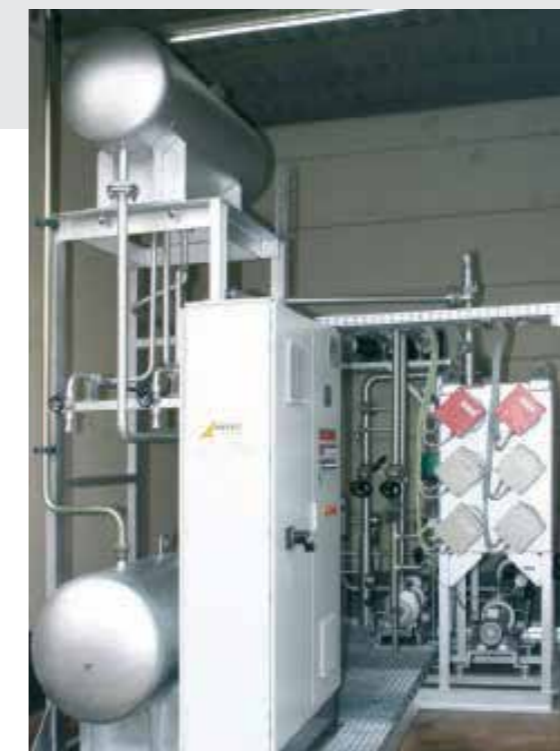
Electric heater with an output of 150 kW with six heating elements for exact regulation of capacity
