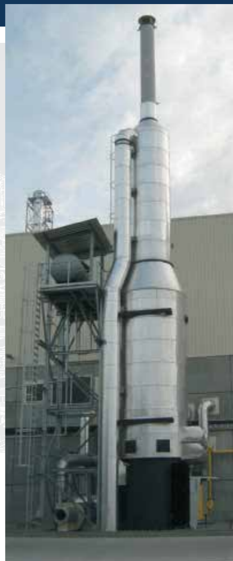
Heater in up-firing layout, capacity: 9.6 MW with built-in combustion air preheater and subsequent stack, total height: 25 m, heating of a particle-board press (Romania)
