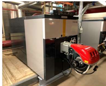
Hot Water Boilers
