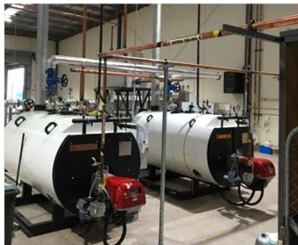
Low Hazard Boilers
