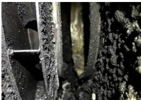
Excessive Waste Material Build Up on ID Fan Impeding Airflow
