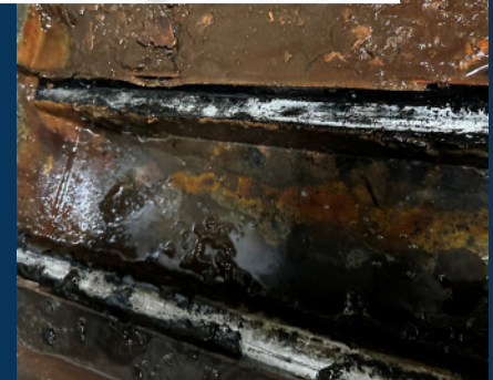
Blocked Check Valve
