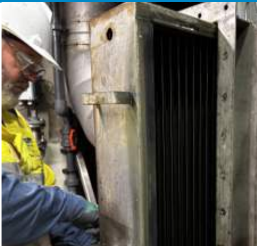
Blocked Chevron Mist Eliminator
