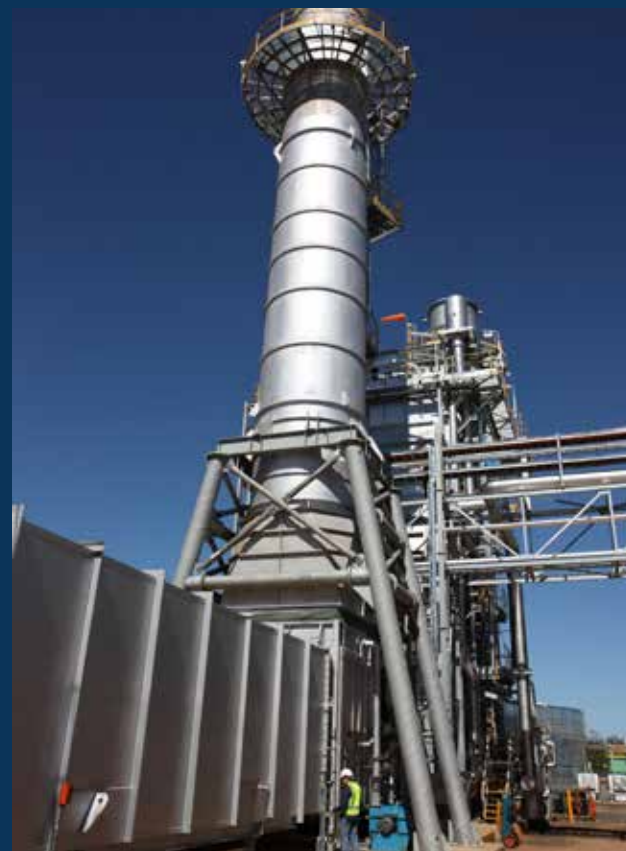
Bypass exhaust system, QLD Australia
