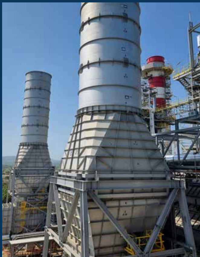
Bypass exhaust system, Colombia
